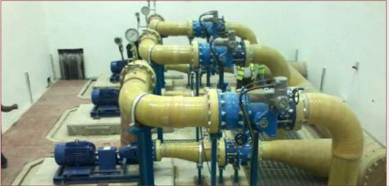
▲ INSIDE THE PUMPHOUSE
